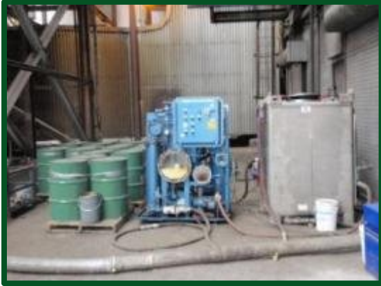
CAN-AK vacuum distillation unit and holding tote.
