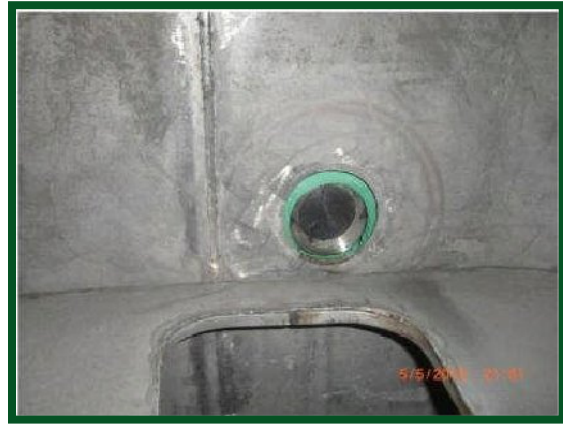
Guillotine 30 Reservoir, 600 USG, after.
