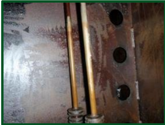
Guillotine 30 Reservoir, 600 USG, before.
