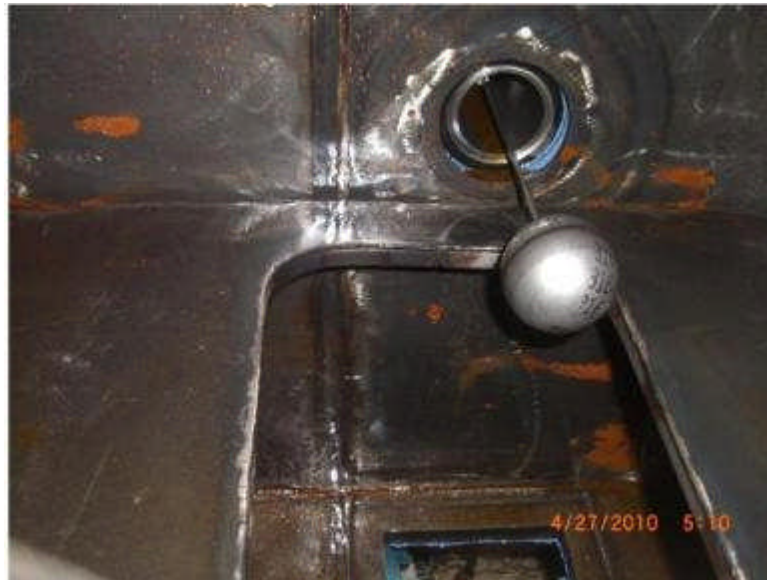
Internal of 60 gallon reservoir before chemical flush
