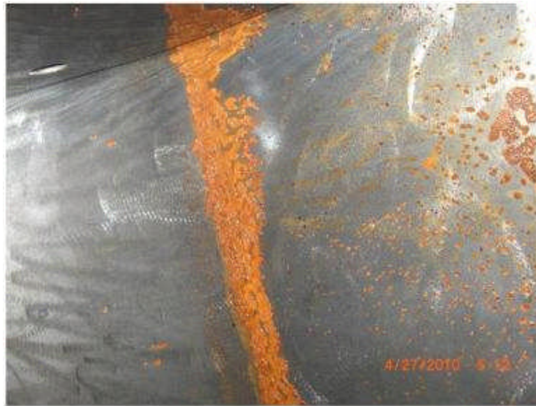
Internal of 60 gallon reservoir before chemical flush
