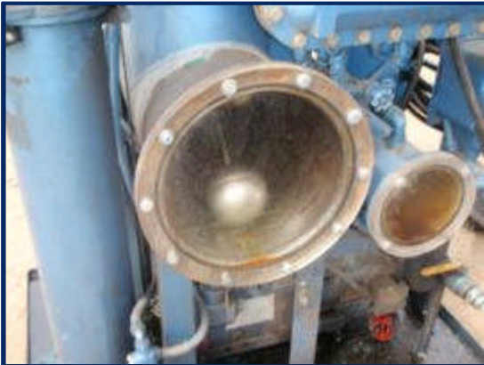
Fluid Purification Equipment being staged
