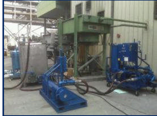
Flushing Equipment in line with system and hold tote
