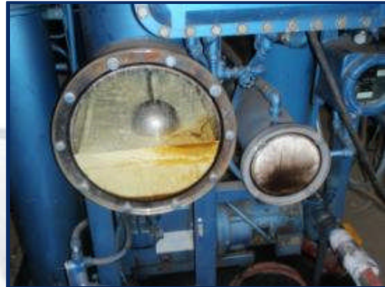
Fluid Purification Equipment in line with system
