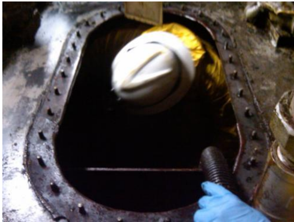
Man inside #1 Dryer Section Reservoir
